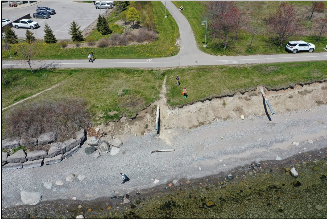
Figure 26. Infrastructure exposed along the Ajax waterfront. Source: TRCA, 2021.
