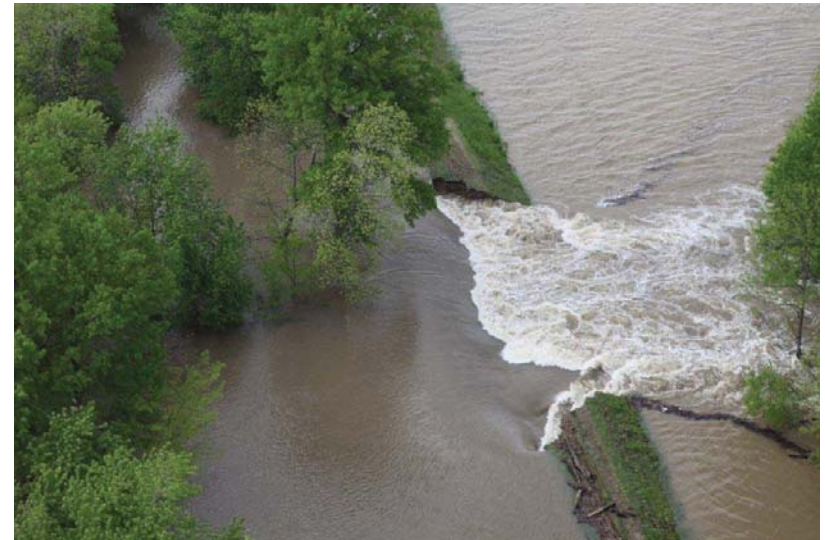
Example of a dyke failure
