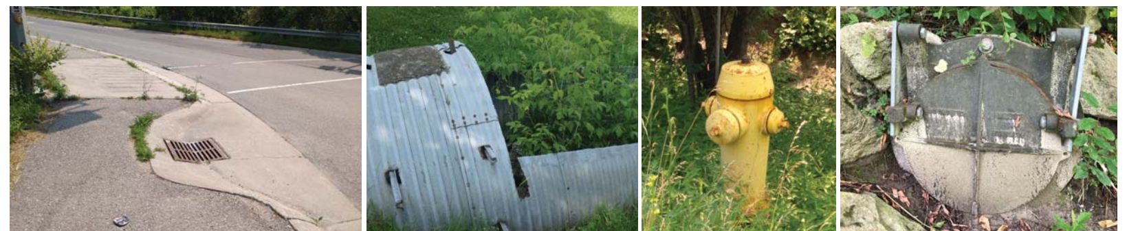
Utilities and drainage infrastructure
