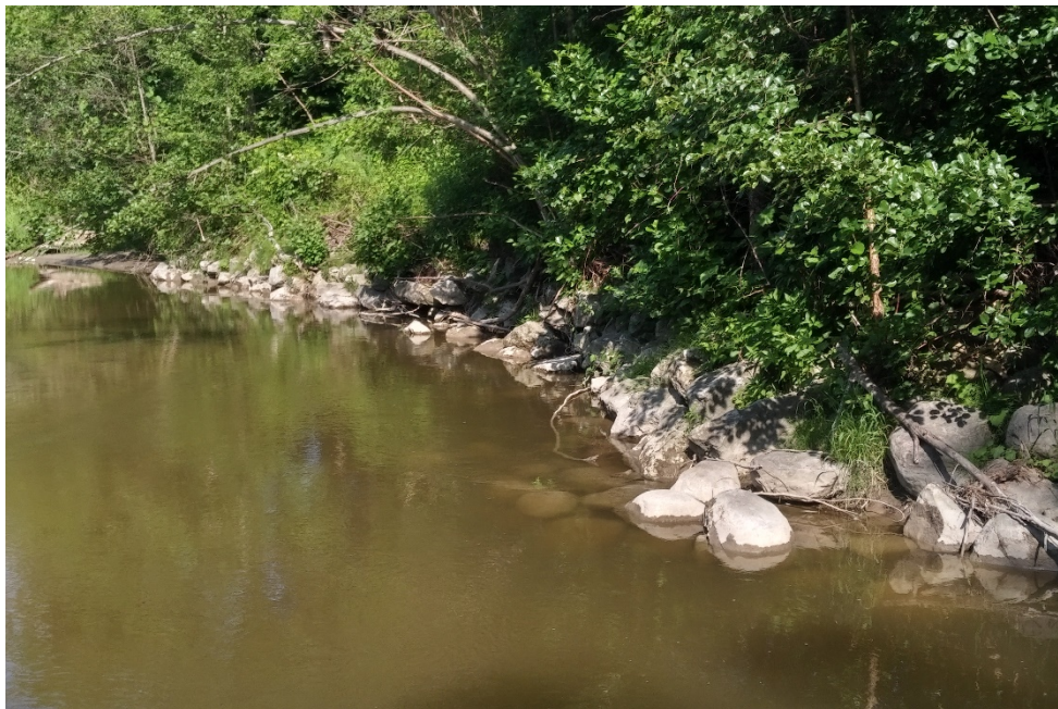
M6-Wet Slope Rip Rap Buttress - Pickering Dyke Wet Slope Approximately 220 m East of Brock Rd
