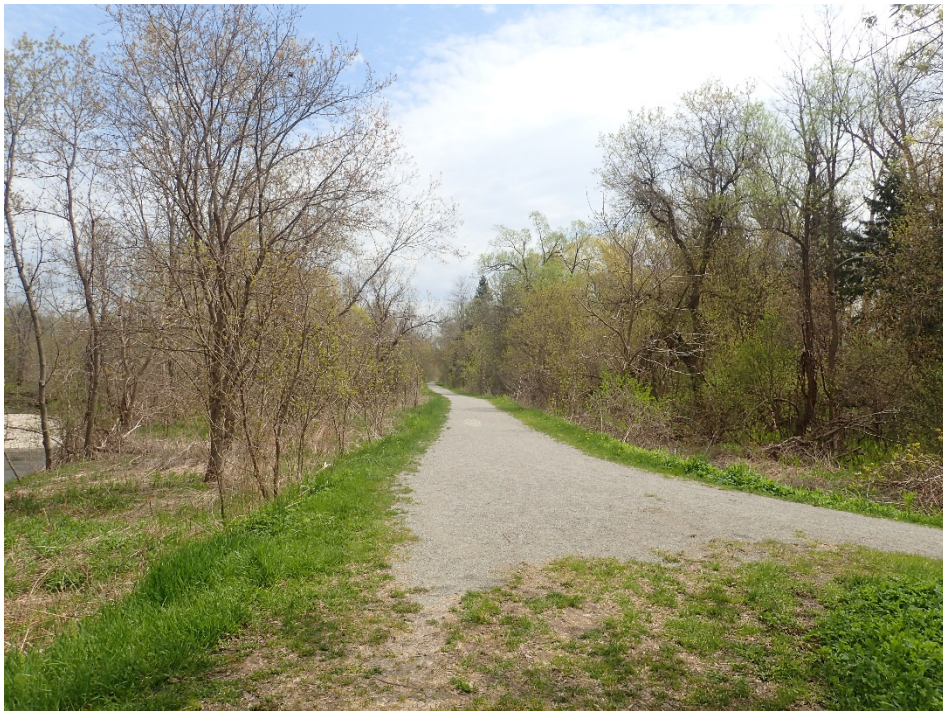
M8 - Pickering Dyke at End of Walking Trail – Trail on Dyke Crest Typical from 400 m to 750 m East of Brock Rd
