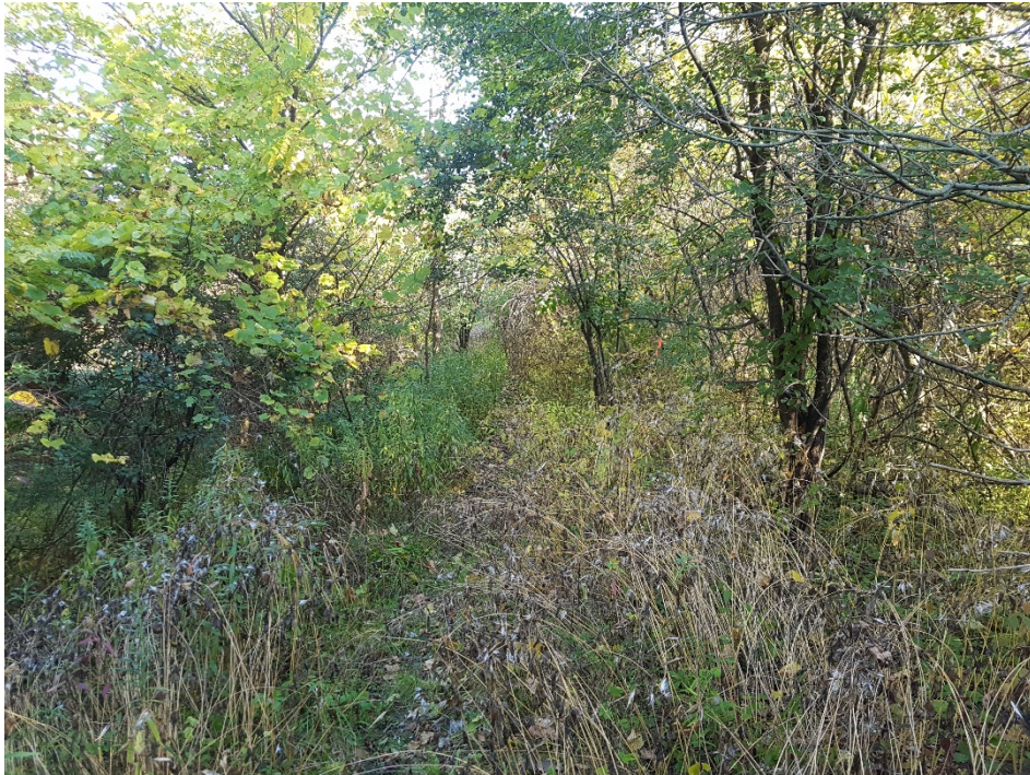
M19 - Ajax Dyke North of Trans Canada Trail Overgrown Vegetation
