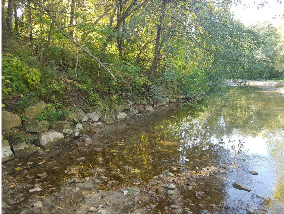
M5-Pickering Dyke Wet Slope Approximately 250 m East of Brock Rd
