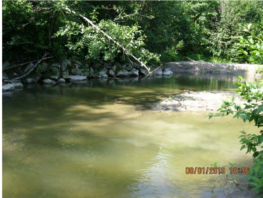
Photo 7. Looking upstream at the boulder revetment (left) and large sand deposit (centre and background)
