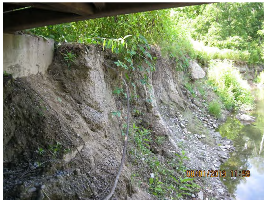
Photo 8. Actively eroding south bank of Duffins Creek (M11) in front and upstream of a pedestrian bridge abutment (looking upstream)
