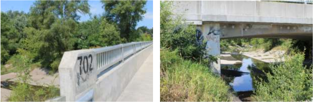
Figures 37 & 38: (left) View of west parapet wall and railing, (right) View of east elevation abutment, wingwall, and soffit from channel embankment (Source: MHBC, 2019)
