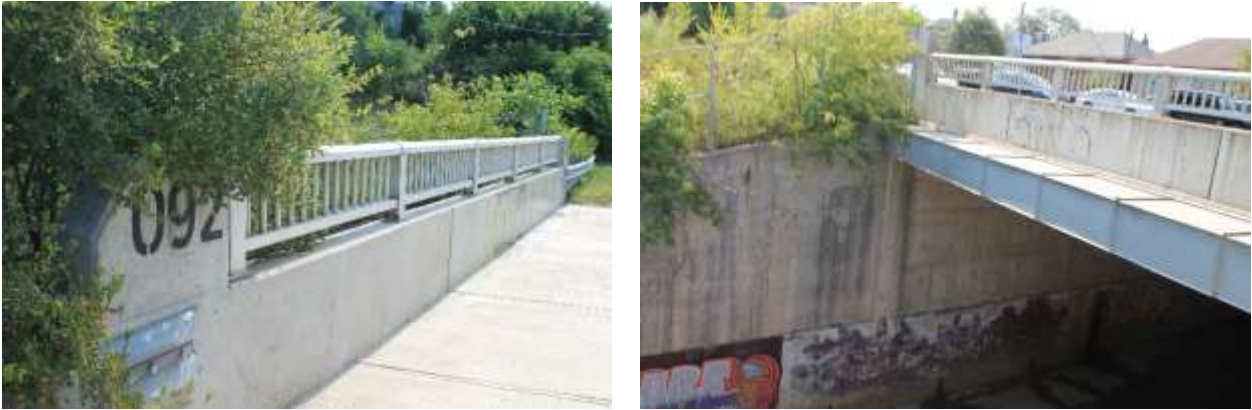
Figures 29 & 30: (left) View of parapet and railing looking north-east from intersection of Weston Road and Black Creek Drive (right) View of northeast retaining wall, soffit and barrier exterior (Source: MHBC, 2019)
