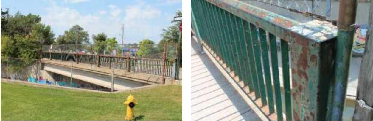
Figures 35 & 36: (left) View of north elevation of bridge railing and soffit, from Humber Boulevard, (right) Detail view of Galvanized steel post and panel railing (painted green, evidence of corrosion) (Source: MHBC, 2019)
