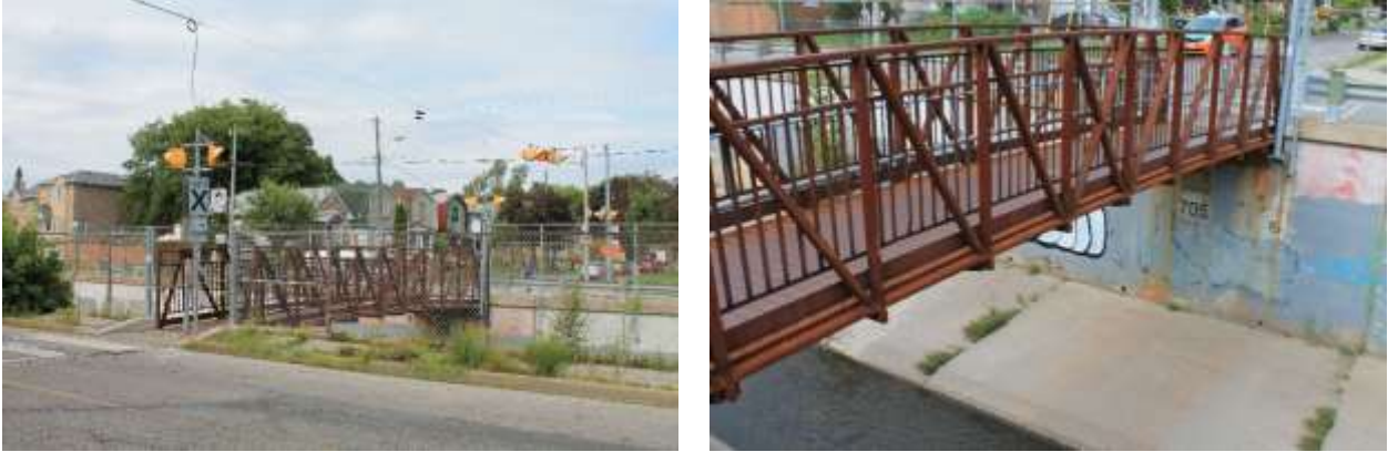
Figures 31 & 32: (left) View of north elevation of truss and approach (right) View of west abutment and retaining wall, north elevation of truss and railing. (Source: MHBC, 2019)
