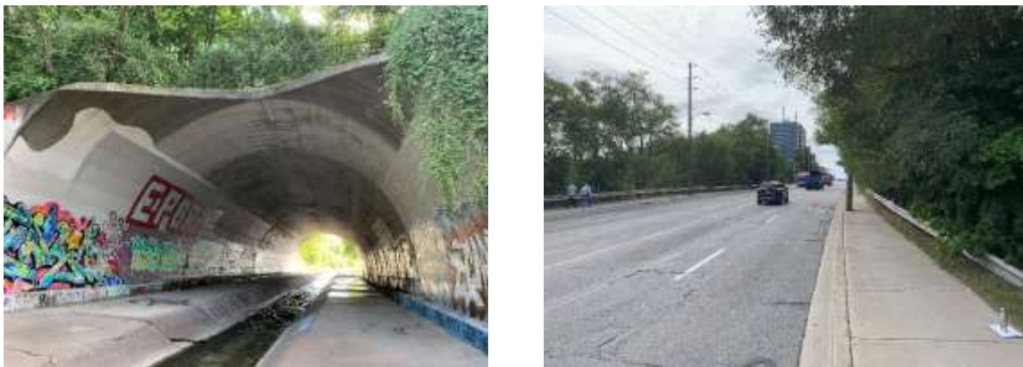
Figures 39 & 40: (left) View of barrel inlet, looking east (right) View of Jane Street looking south over culvert, (Source: MHBC, 2019)
