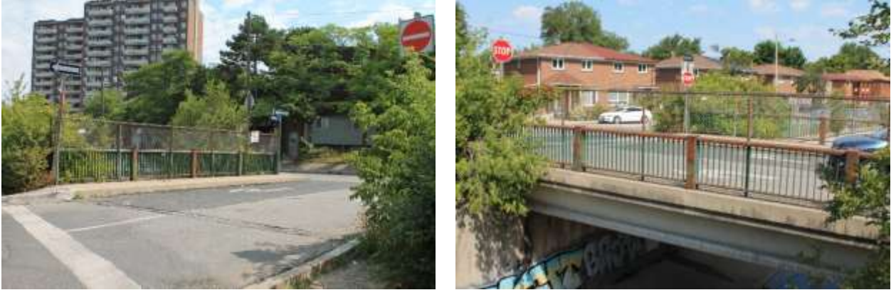
Figures 33 & 34: (left) View of west approach asphalt surface, sidewalk, railing, and chain-link fence, (right) View of south elevation railing, abutment, and soffit (Source: MHBC, 2019)
