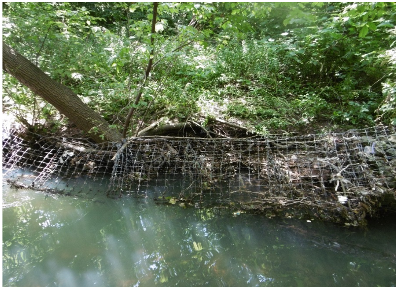
Description of Photo: Failed gabion on left bank facing DS
