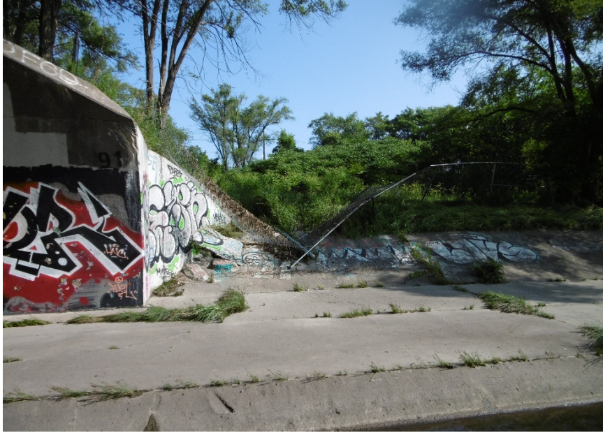
Description of Photo: Damaged Fence on upstream side
