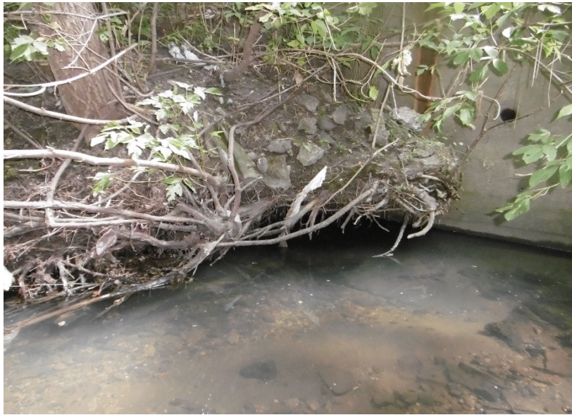
Description of Photo: Severe erosion
