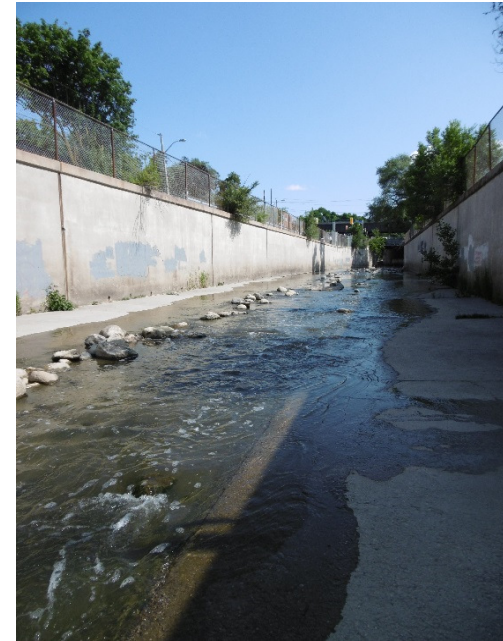
Description of Photo: Displaced rocks on downstream side
