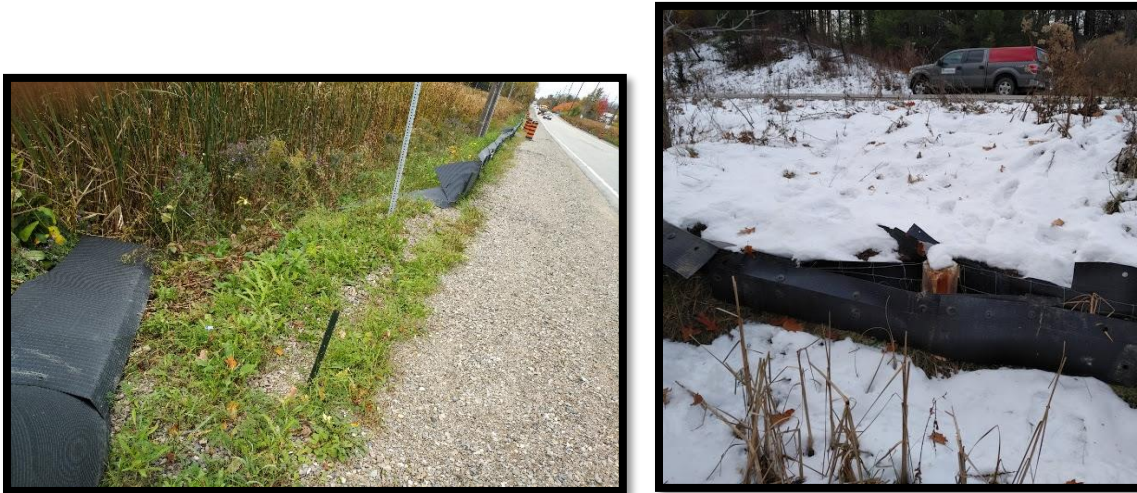
FIGURE 24. DAMAGE TO TEMPORARY FENCING AND PERMANENT FENCING ALONG HEART LAKE ROAD IN 2018.
