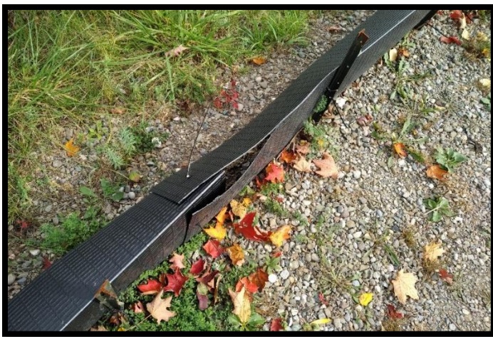
FIGURE 9. TEMPORARY WILDLIFE DIRECTIONAL FENCING WITH MINOR DAMAGE.
