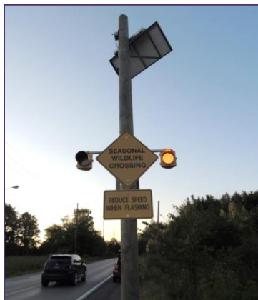
Figure 25: CoB solar-powered, flashing seasonal wildlife crossing sign
