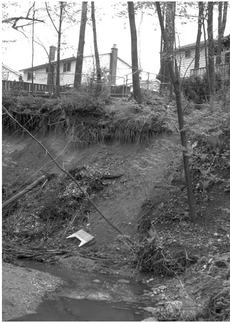
Erosion along Highland Creek
