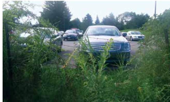
1. Fence damage along boundary with Meadowbrook Golf & Country Club
