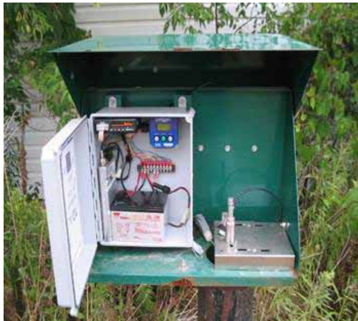
Figure 30: PGMN well with telemetry equipment and dedicated pump installed
