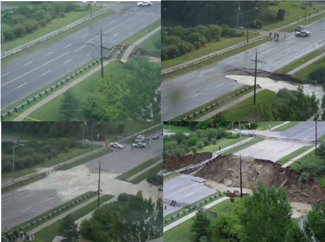
Figure 42: Finch Avenue culvert failure August 19 th , 2005 Toronto, Ontario, >125mm in 1 hour.
